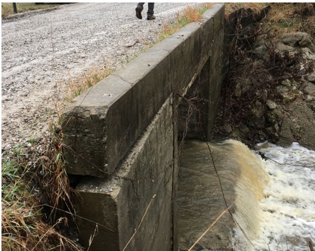
Damaged culvert before replacement
