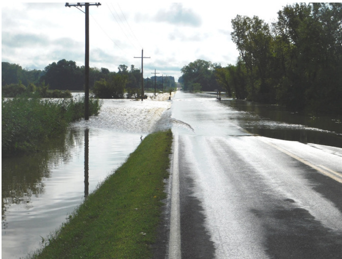
N 1000 RD flooded July 2017
