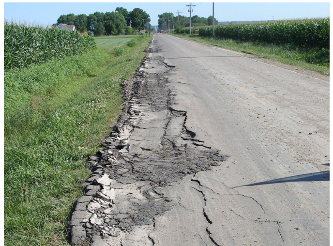
Pavement damage Route 9
