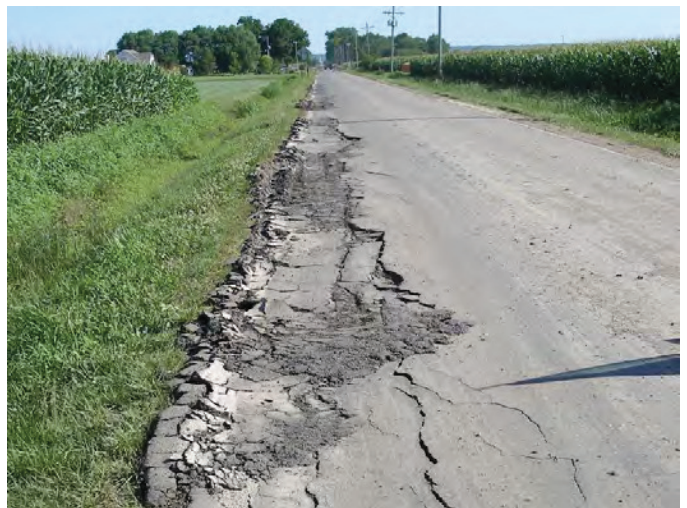
Pavement damage Route 9
