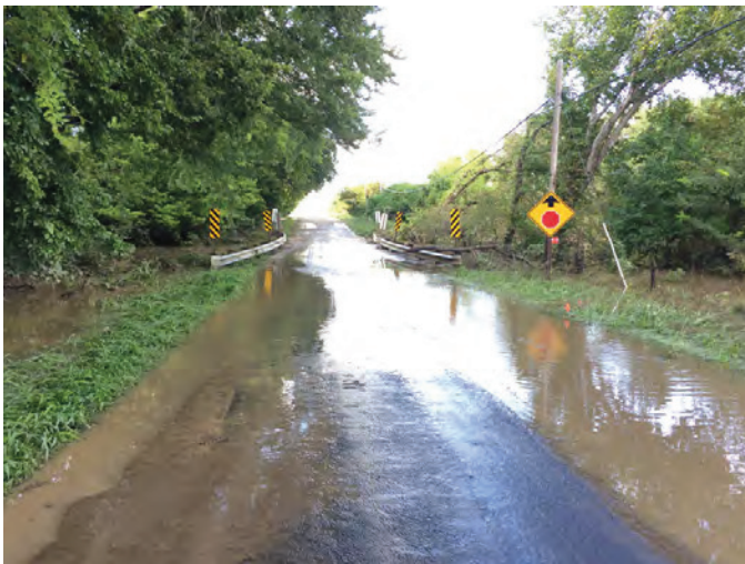
Existing roadway flooded July 2017
