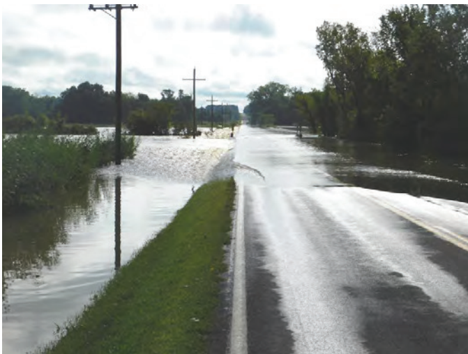
N 1000 RD flooded July 2017
