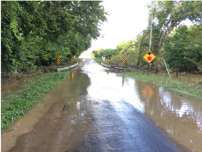
Existing roadway flooded July 2017
